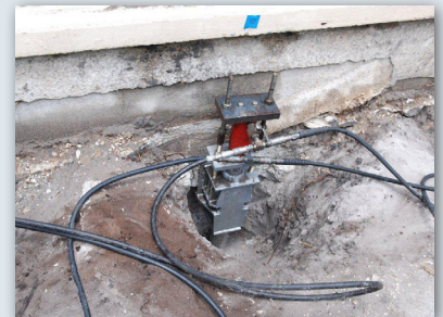
Hydraulic cylinders connected to brackets
