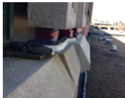
Plastic shims at separation
