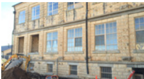
Southeast corner of wing experiencing settlement
