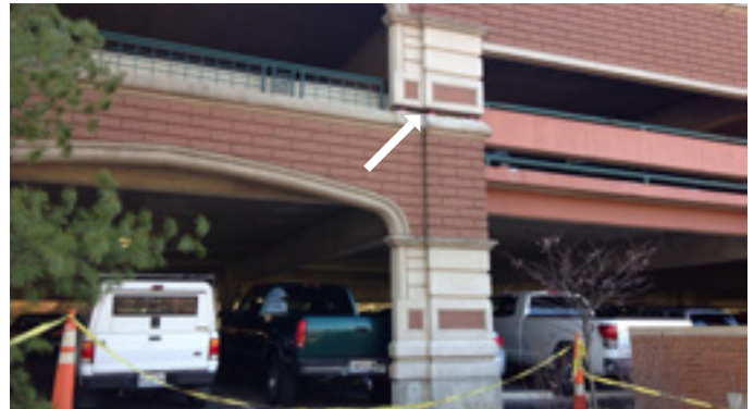
Settled façade; separation
