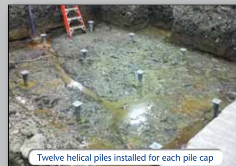
Limited access and working space within existing building
