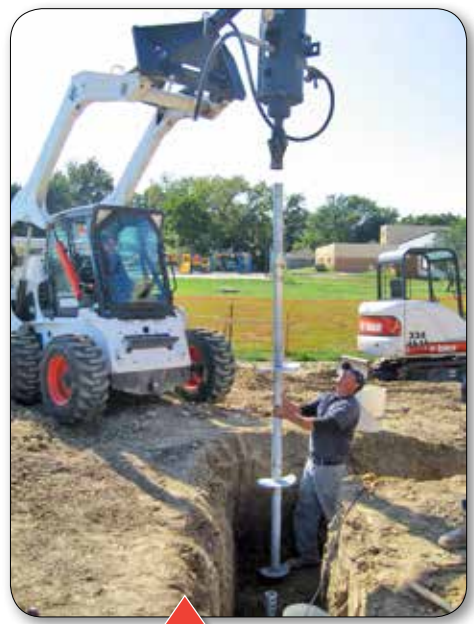
Helical piles to support foundations of a high school weight room addition
