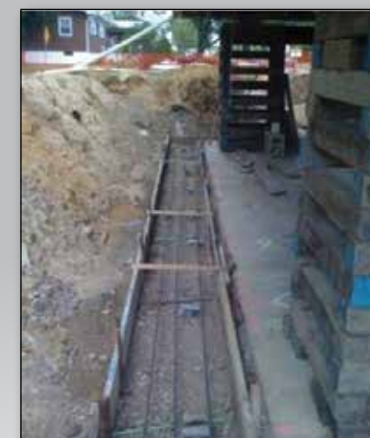
Rebar is placed over installed new construction piers. The footing is ready for concrete.
