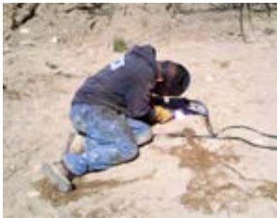
Piles cut to design elevation and new construction brackets tack-welded in place
