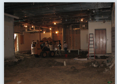
Piles are installed in limited access areas within the building using small construction equipment
