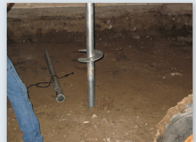
Helix lead sections are advanced through hard, dry to damp fill soil layers
