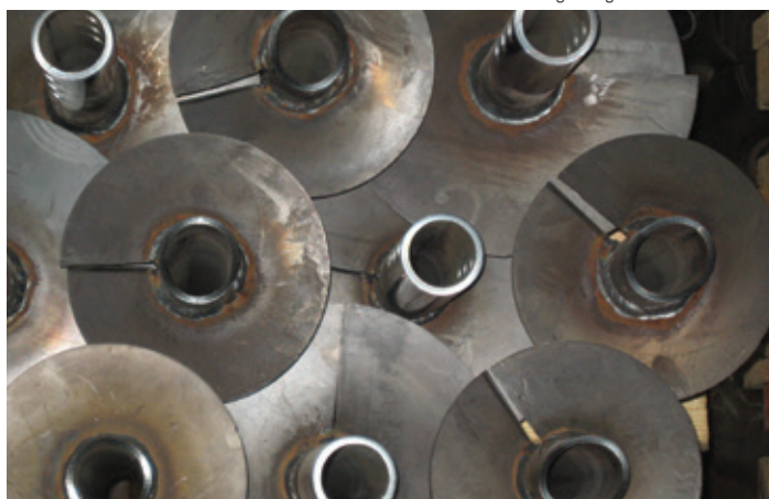
Black steel beginning to show corrosion
